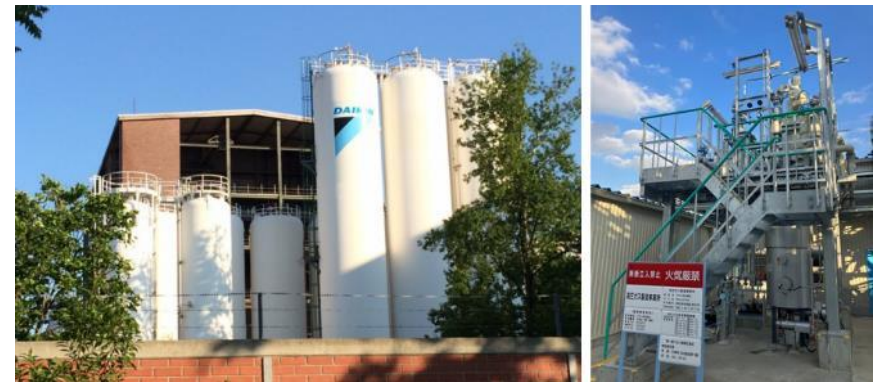
A destruction and reclamation plant began operation in Germany in 2023 (left) A new fluorocarbon reclamation facility has been established at the Yodogawa Plant (right)
