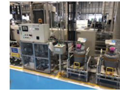
Recovering refrigerant in the production process
