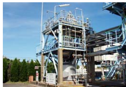
Destruction facilities for recovered fluorocarbon
