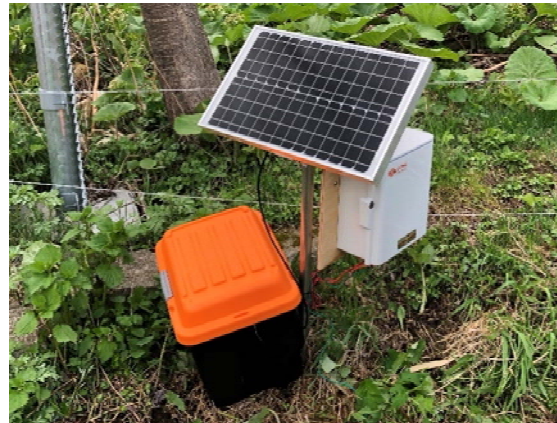
Photo 2-8. EfMos installed (remote monitoring system)
