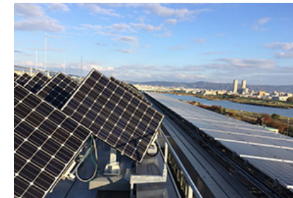
Solar power generation system has panels that move to track the sun's position (at TIC)
